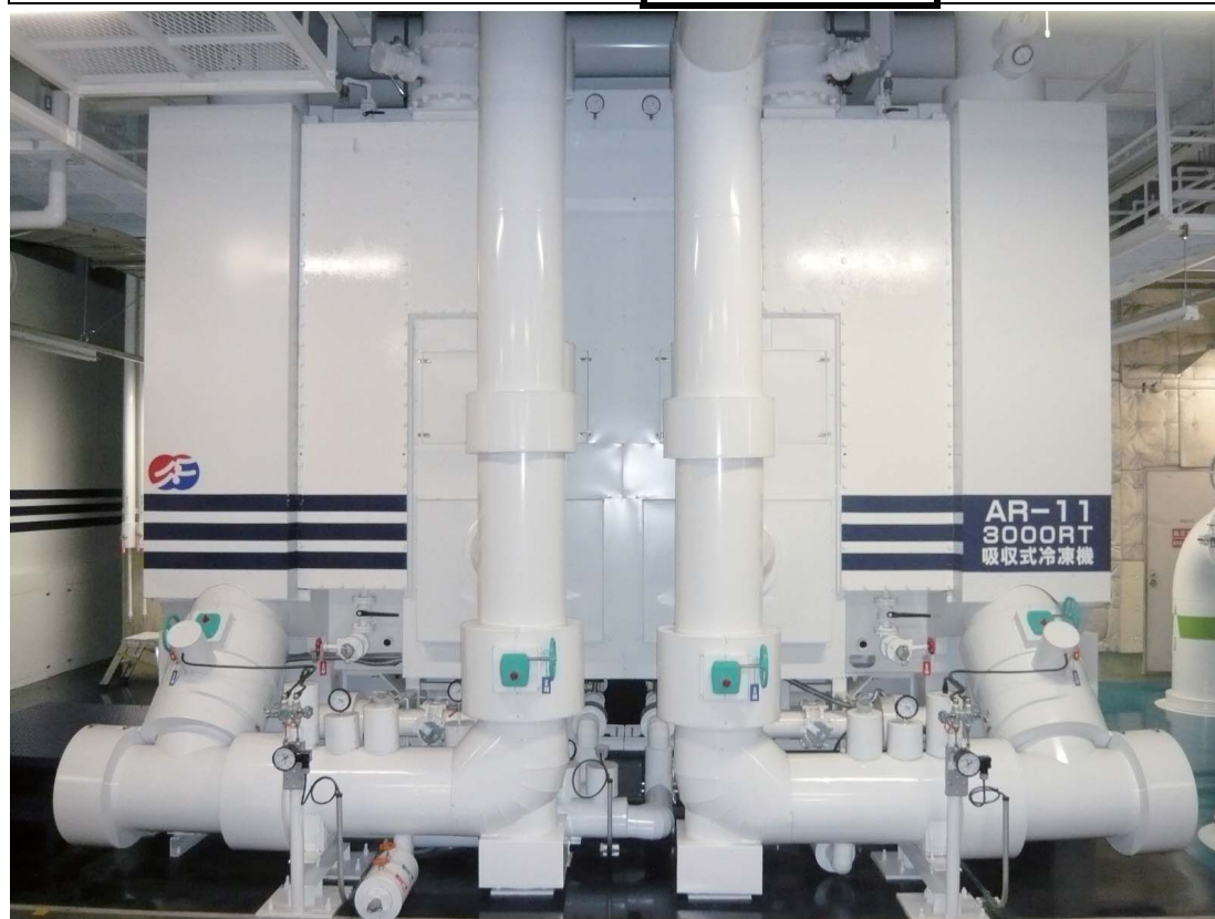
New 3,000RT absorption chiller units installed at the Central Plant in June 2015
