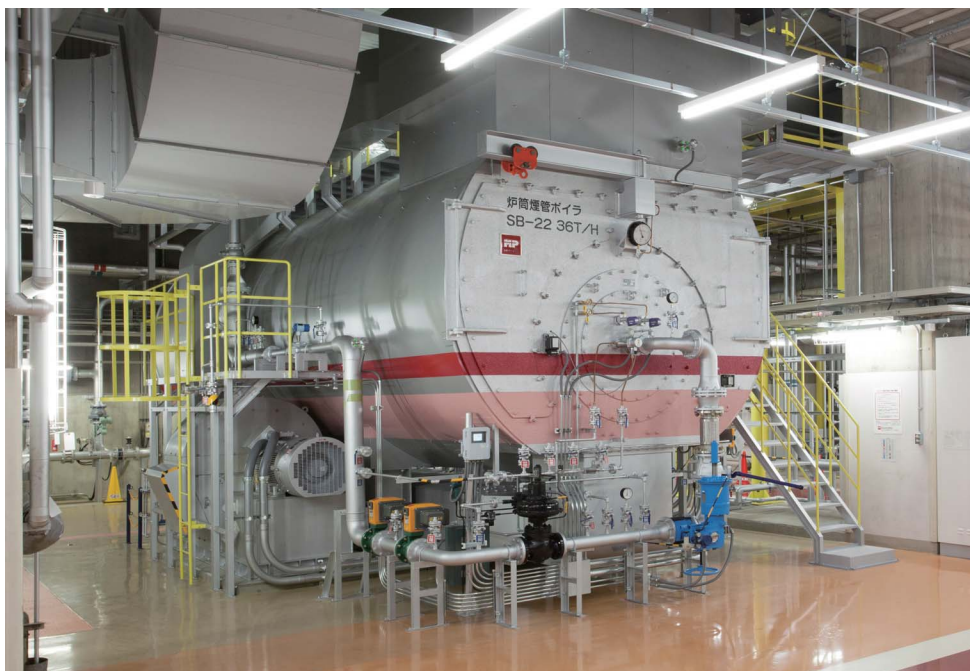
The additional 36 t/h flue and smoke tube boiler installed in the No. 2 Plant in September 2014
