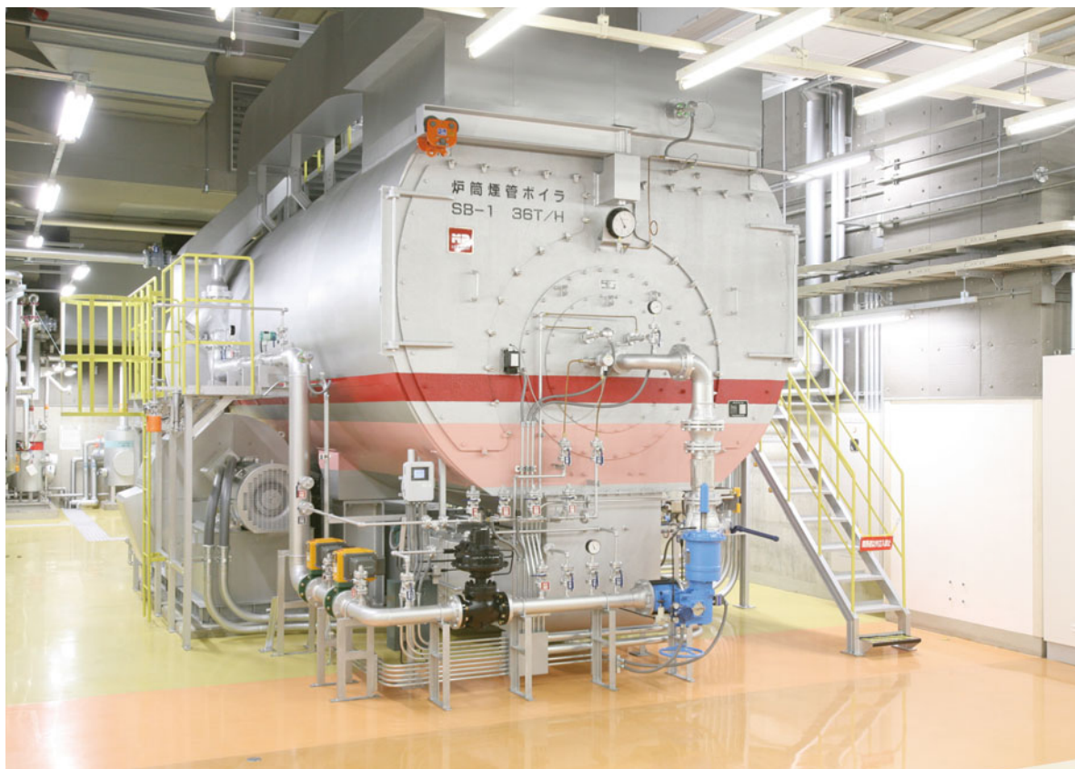
The 36 t/h flue and smoke tube boiler newly installed in the No.2 Plant in December 2010
